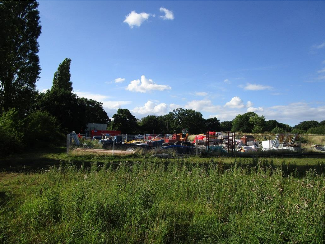
Photo 9 – the construction site compound at the west of the site, viewed from the south-east
