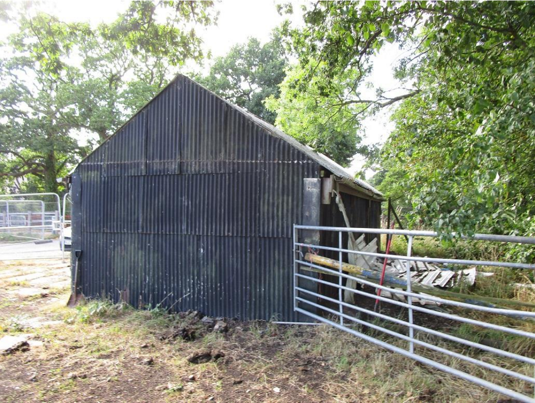
Photos 7 and 8 – The corrugated metal-clad stable block, with several birds nests inside
