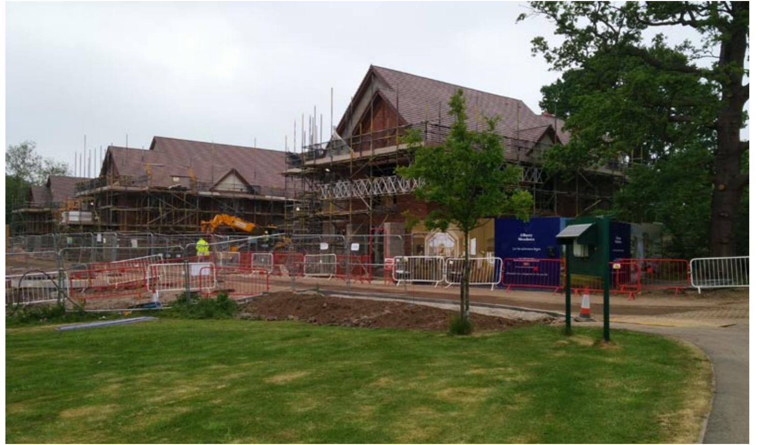
Photo P10 - Albany Meadows Care Village under construction which abuts the western boundary of the proposed allocation site
