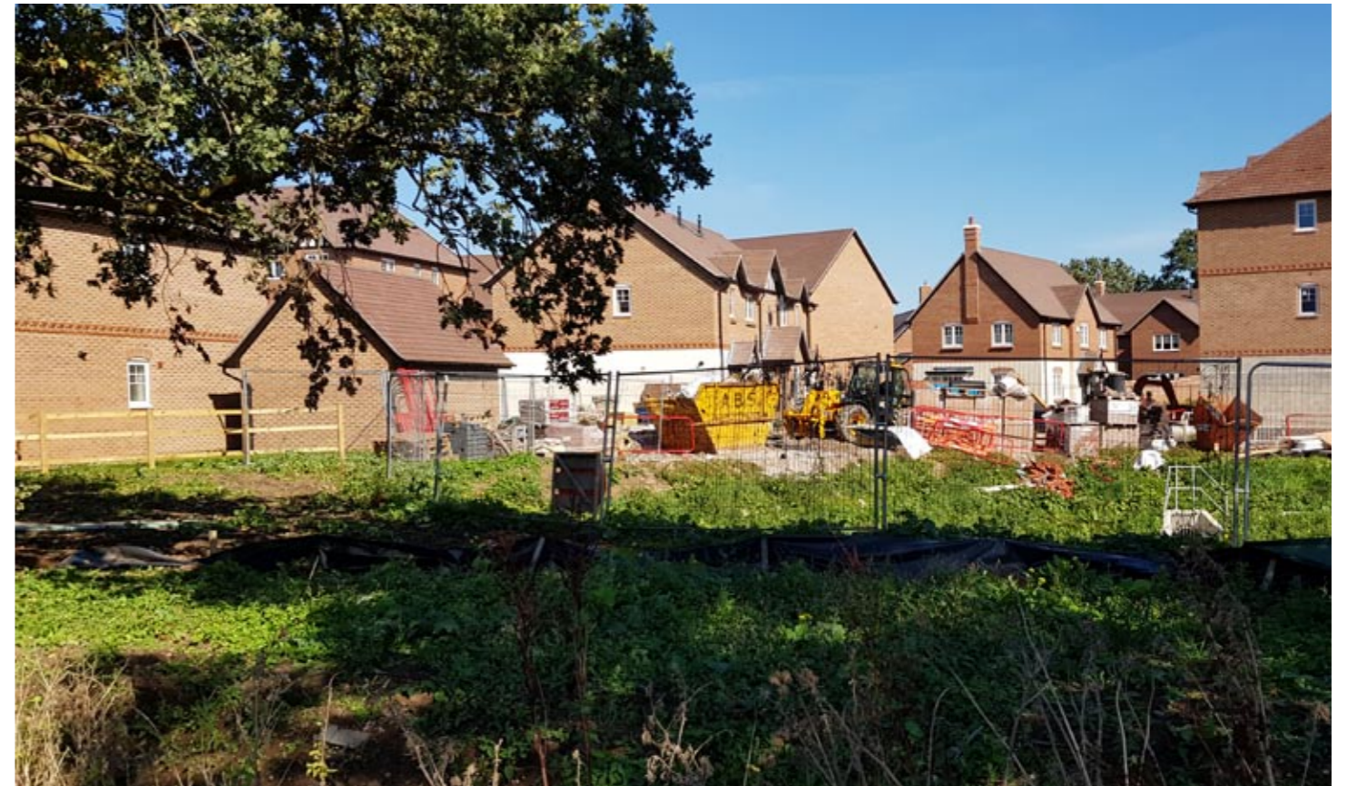
Photo P8 - New residential development under construction adjacent to Kenilworth Road east of the proposed allocation site
