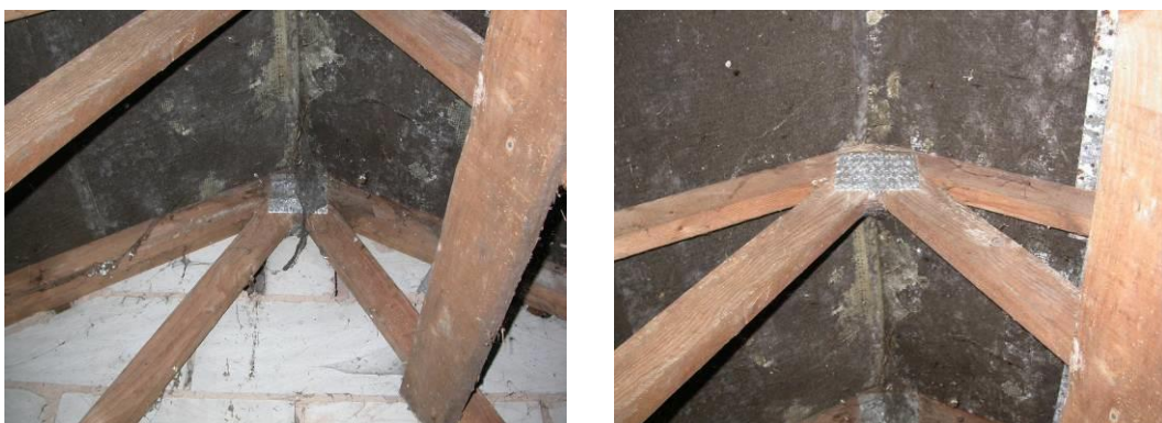
Figs. 33 & 34 Cobwebbed roof void
