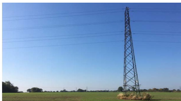
Existing overhead lines on the east of the site
